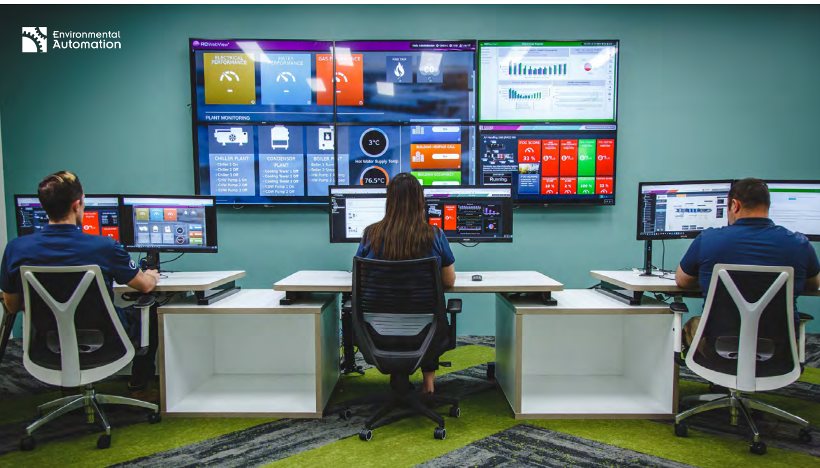
The EA Plus team at Environmental Automation's national monitoring center in Kingsgrove, NSW, delivers analytics and optimization strategies with reliable data using RC-Reporter software from Reliable Controls.
